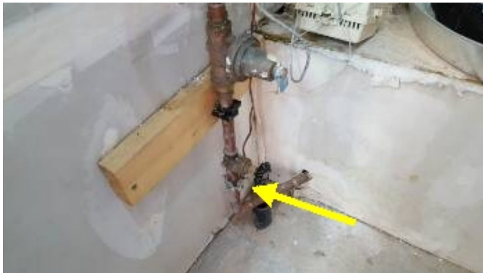
In water heater closet off the garage
